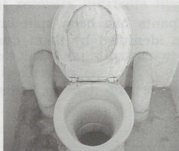
Enviroloo at the KDC offices
